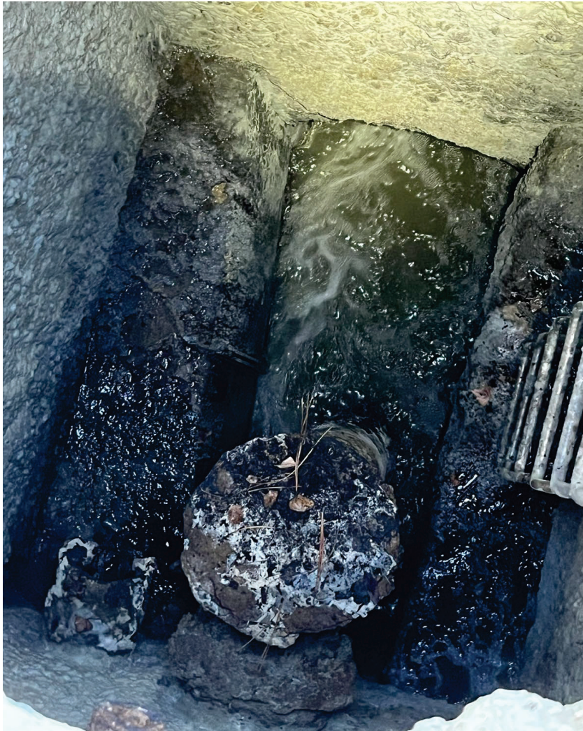
Found Condition – Major Corrosion
