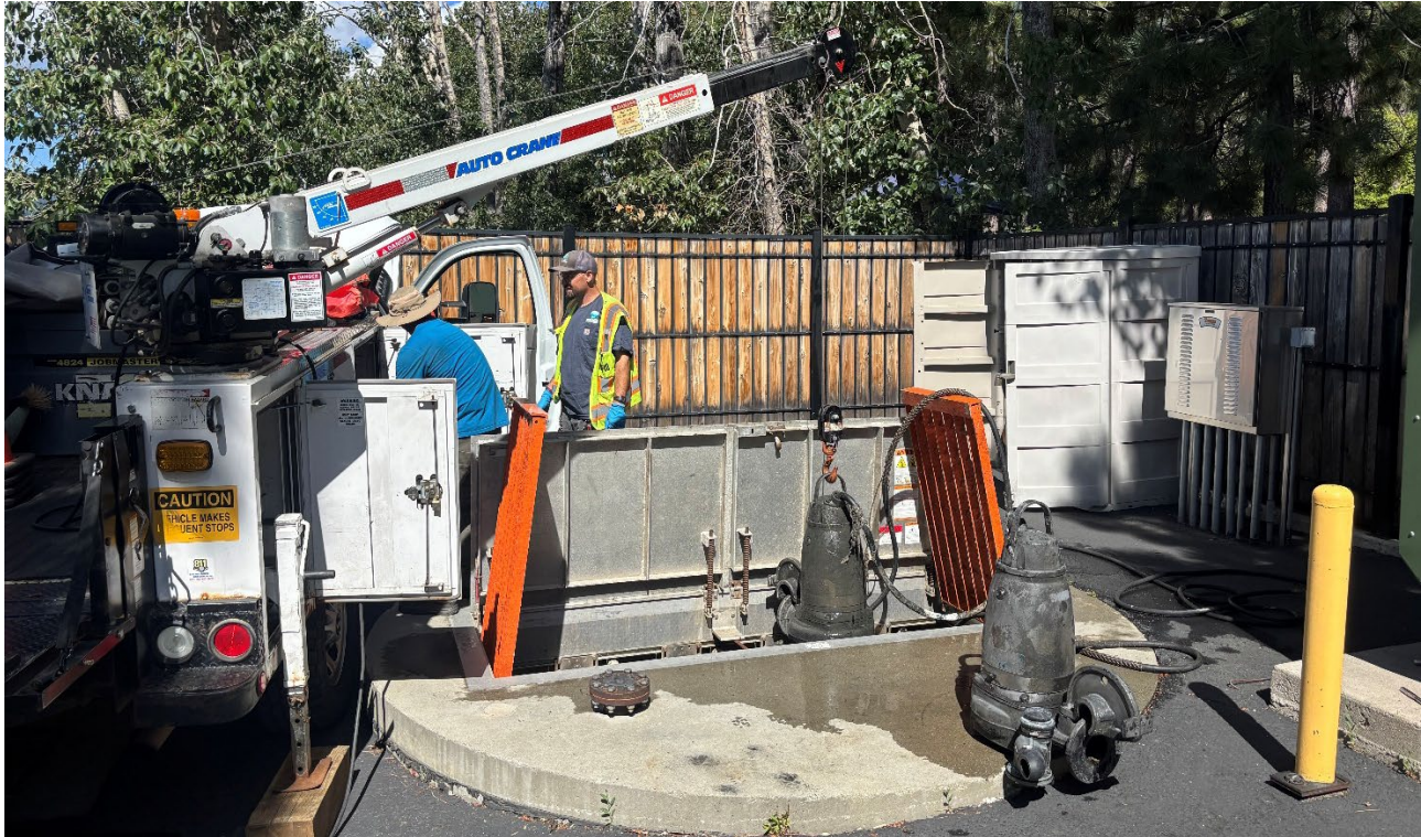
Annual Secline Main Station wastewater pump inspection and service.
