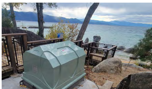
New station at S-1
