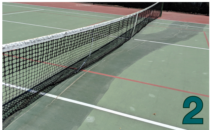
Surface Cracking Along Net
