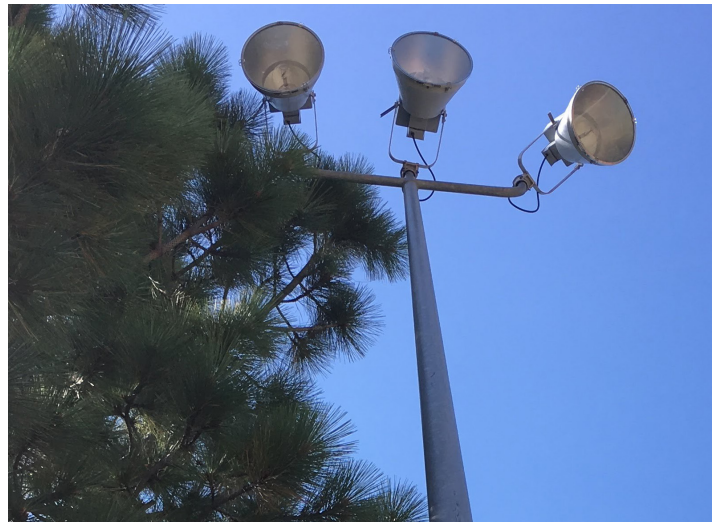
South Court Lighting
