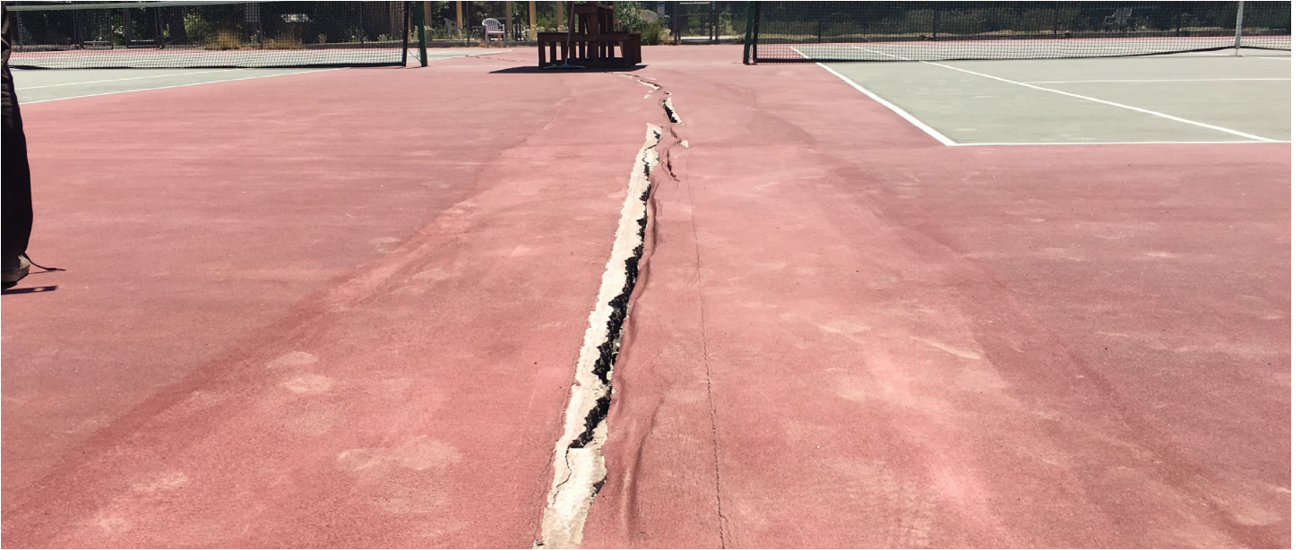
Image 5: Significant cracking through south tennis courts
