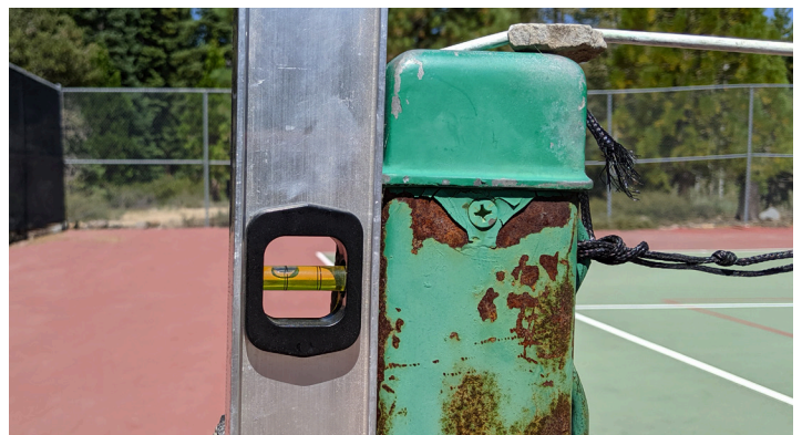
Image 10: Net posts were rusted and bent
