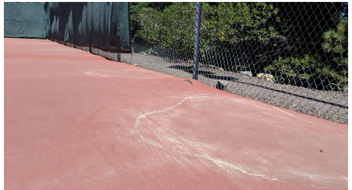
Image 6: Areas of ponding evident on surface
