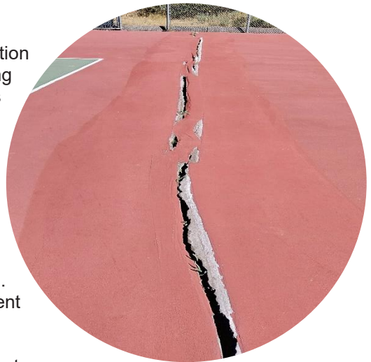
Photograph 1: Previously patched large shrinkage crack, note vegetation growing through the center.
