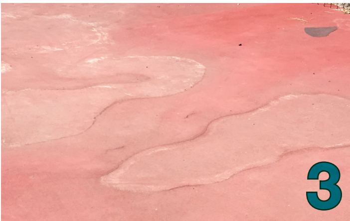
Evidence of Ponding on Surface
