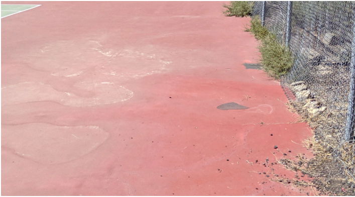
Image 3: Surface bulging and cracking along perimeter
