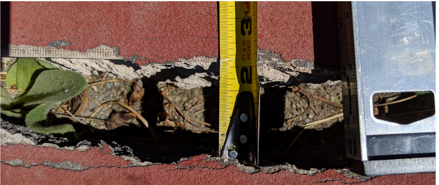
Image 6: Significant cracking through south tennis courts
