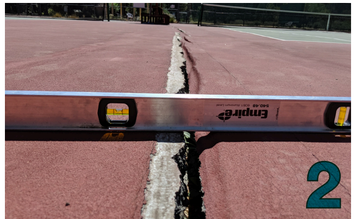
Court Surface Cracking
