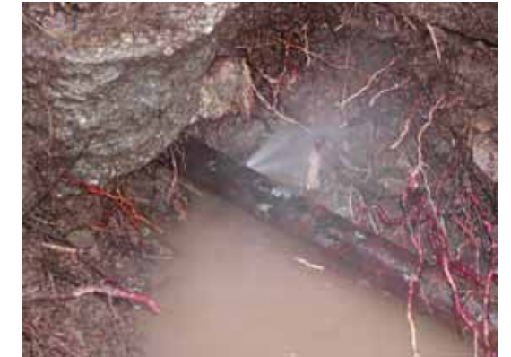
An old, leaky and undersized water pipe.
