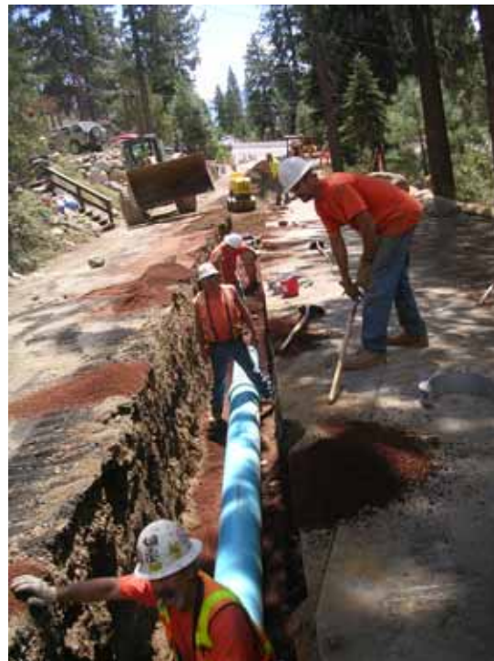
Installation of the new water pipe on Beaver Street, the 2007 Capital Improvement Project.
