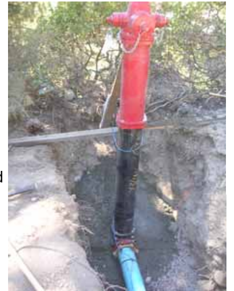
Fire hydrant installation will be a result of water system improvements. This new plug is being installed as part of the 2007 Beaver Street Project.
