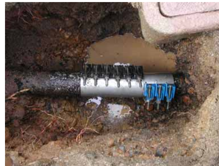
Many water lines in the District are old and have repair clamps installed that have fixed prior leaks.
